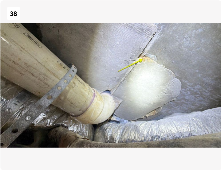
Staining was observed around portion of the deck patching material.
