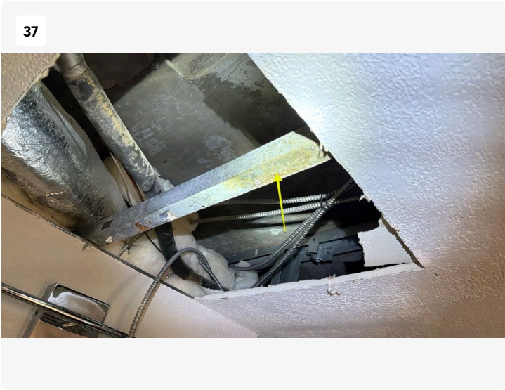
Staining was observed on portions of the ceiling framing.
